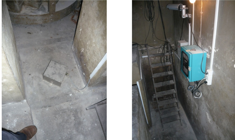
Figure 3 – Photographs of the strong-motion station SNES. The sensor (left) is placed on the ground next to NEU. The datalogger (right) is located on the wall and the data can be accessed by a modem connection.
